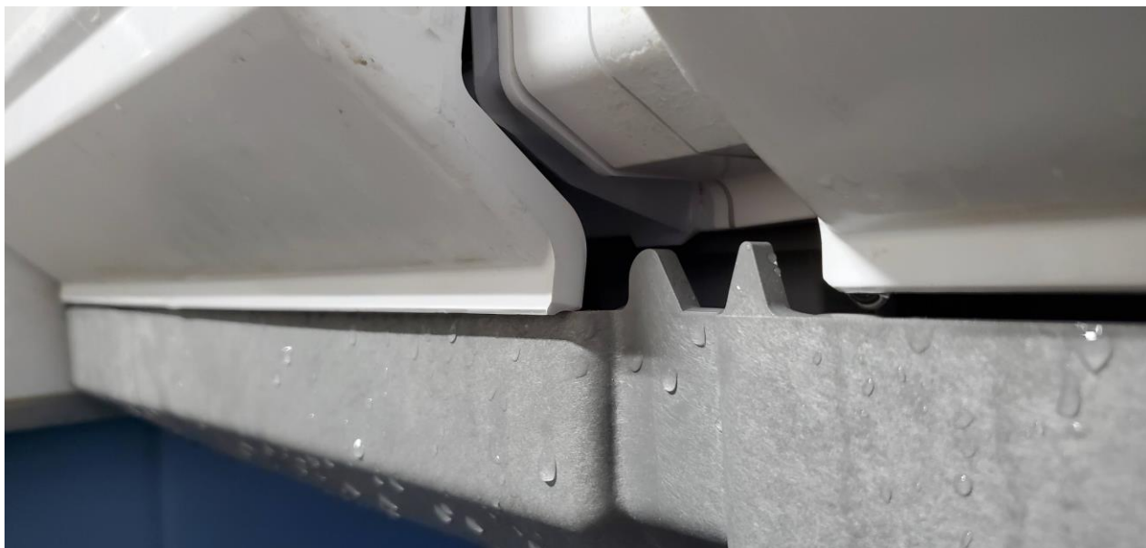
Figure 2: Interference between the sump and curtain when the insert is not installed
